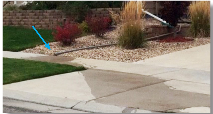
Improper discharge Cut back minimum 10 feet from sidewalk
